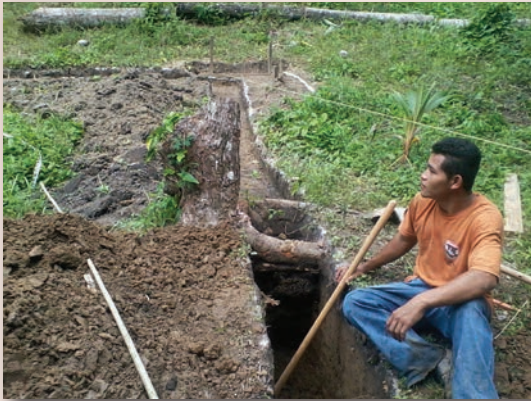
(Above) Sito and many other young men in the community went to work on digging the foundations by hand, for the Give2GiveHope vocational school.
